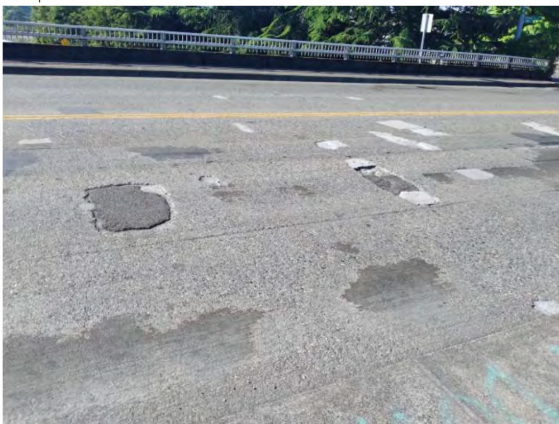
This is the Albro Street bridge over I-5 in Seattle showing deterioration with cracks and pothole patches. Crews will remove large sections of the deck to replace with new concrete.
